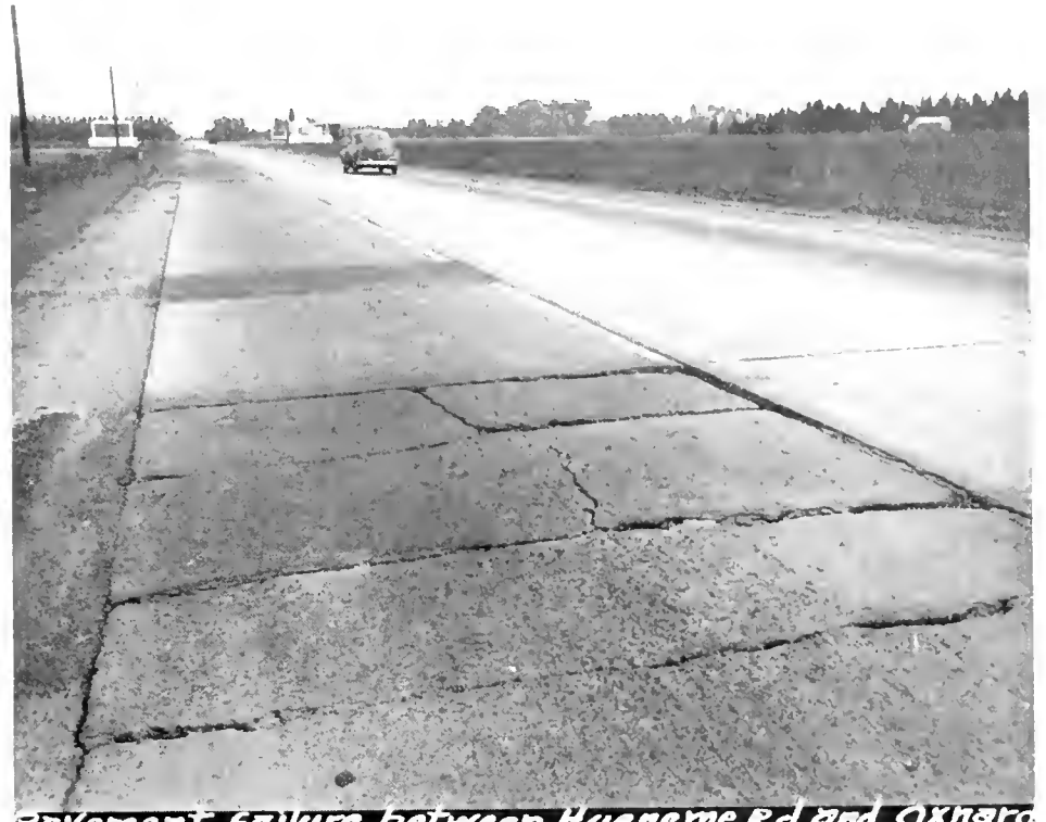
Pavement failure between Hueneme Rd and Oxnard
